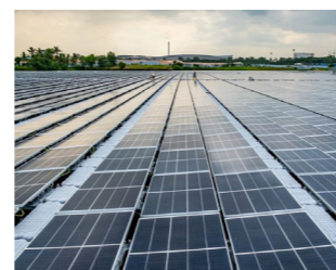
Solar Power Plant
